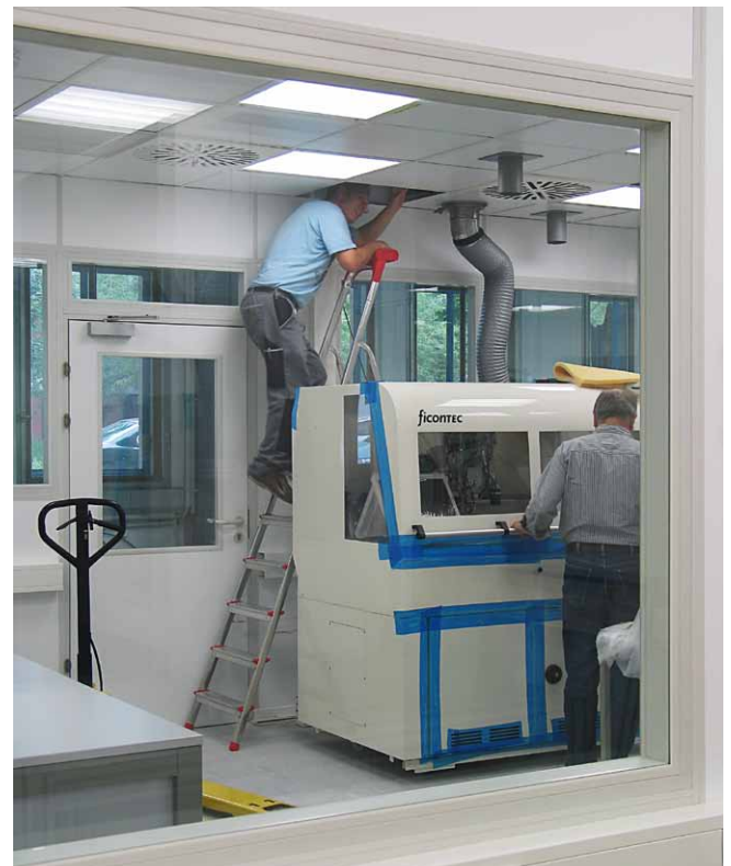
Excellent working conditions after comprehensive construction works at FBH's mounting and packaging area.
